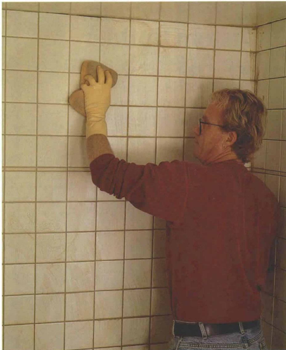
Fine tuning. After packing a wall with grout, use a damp sponge to shave high spots and fill voids.
