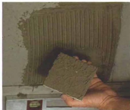
Right trowel. Minimal squeeze-out and complete coverage on the back of this tile denote a properly sized and notched trowel for applying mortar. If mortar had oozed from the edges of this test tile, the author would have switched to smaller notches. This test was done with a \frac{1}{4} -in. by \frac{3}{8} -in. trowel.
