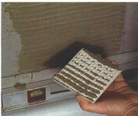
Wrong trowel. Determine the right trowel-notch size by spreading mortar on a small patch of wall. Then, comb the mortar with the trowel and firmly press the tile into the mortar. Pull the tile away and assess the coverage. There shouldn't be any bare spots. This test was done with a \frac{1}{4} -in. by \frac{1}{4} -in. trowel.
