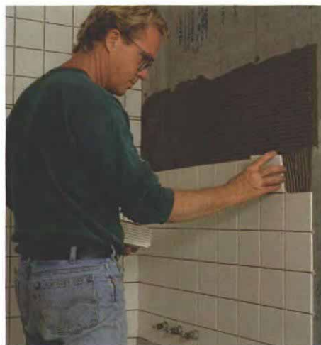
Setting the tiles. With the bottom of the tile resting on spacer blocks, the author tilts each tile onto the mortar and then presses it home.
